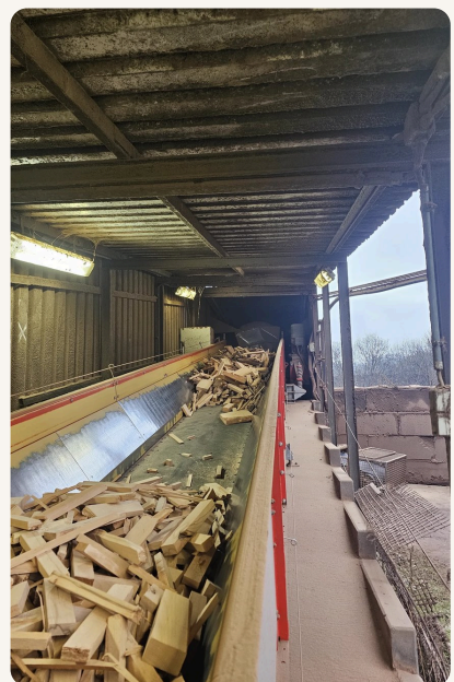
WOOD CHIPS • BIOMASS CONVEYOR
